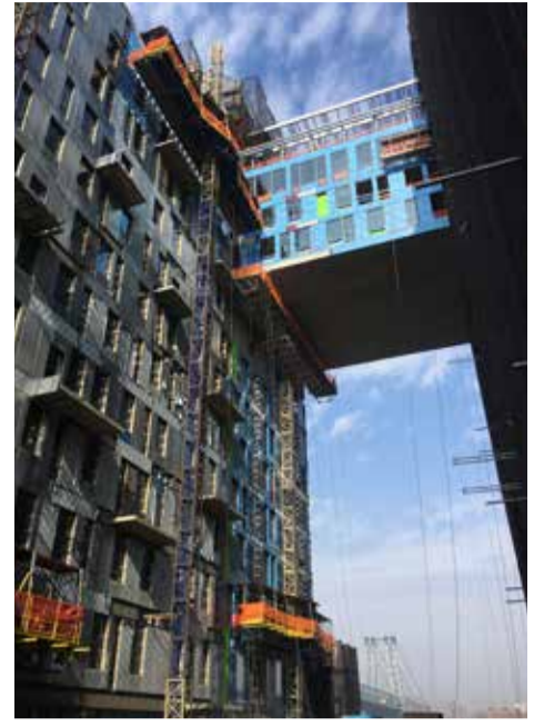
A customised façade system emerges on the lower East Side of Manhattan
