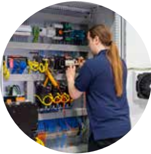
CONTROL SYSTEM DESIGN & MANUFACTURE
